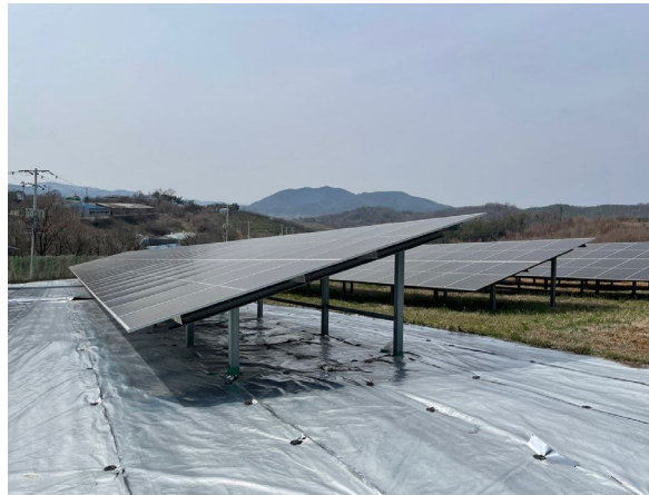
Solar power generation facility
